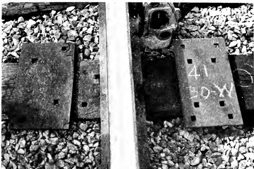
Fig. 8. Middle Portion Section 41, 14-in (1951) Faxon Tie Pad. Bottom: Coated, After 3-years' Service in the Inner Rail of the 5 o Curve
